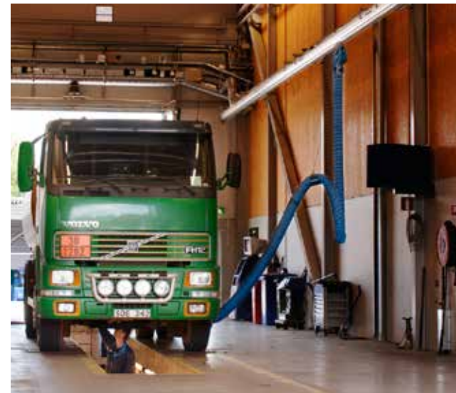
Example exhaust system for vehicle inspection.
